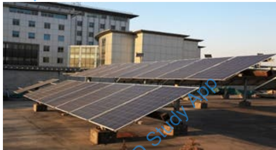
Solar Panels on Roof Top
