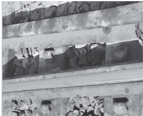
Fig. 7.2 Showing large gap at insert
