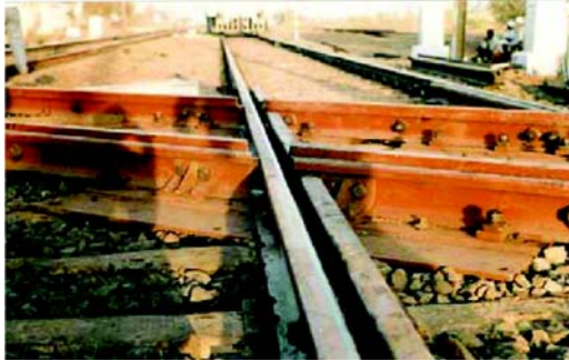
Fig. 3.21 Continuous rail of main line
